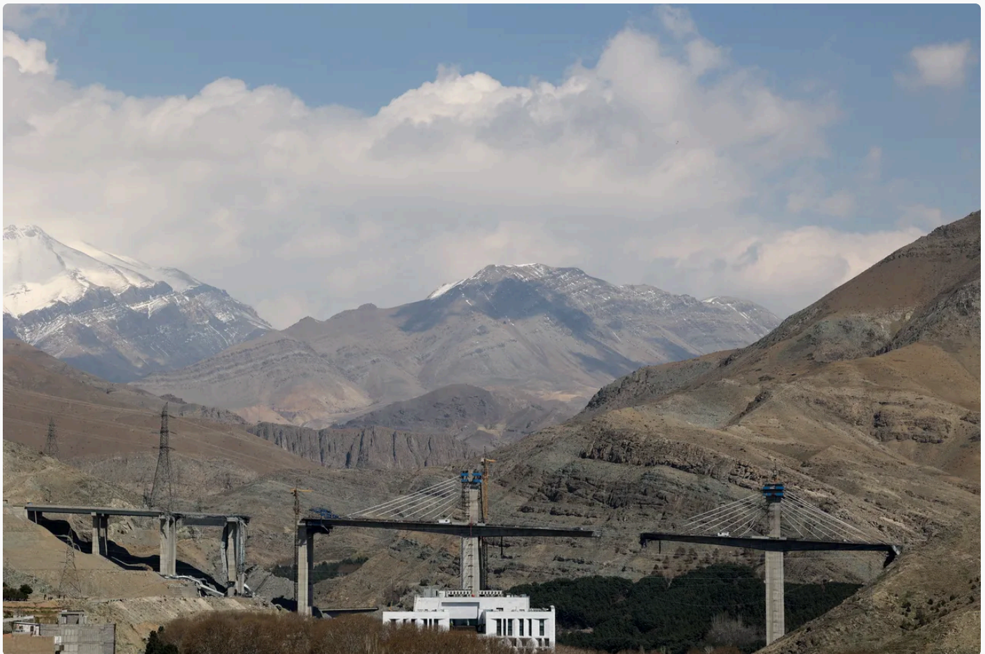
The B1 bridge damaged by a strike, as the US-Israeli war with Iran continues, in Karaj / Reuters
