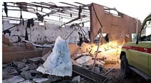
Destroyed facility after the attack
