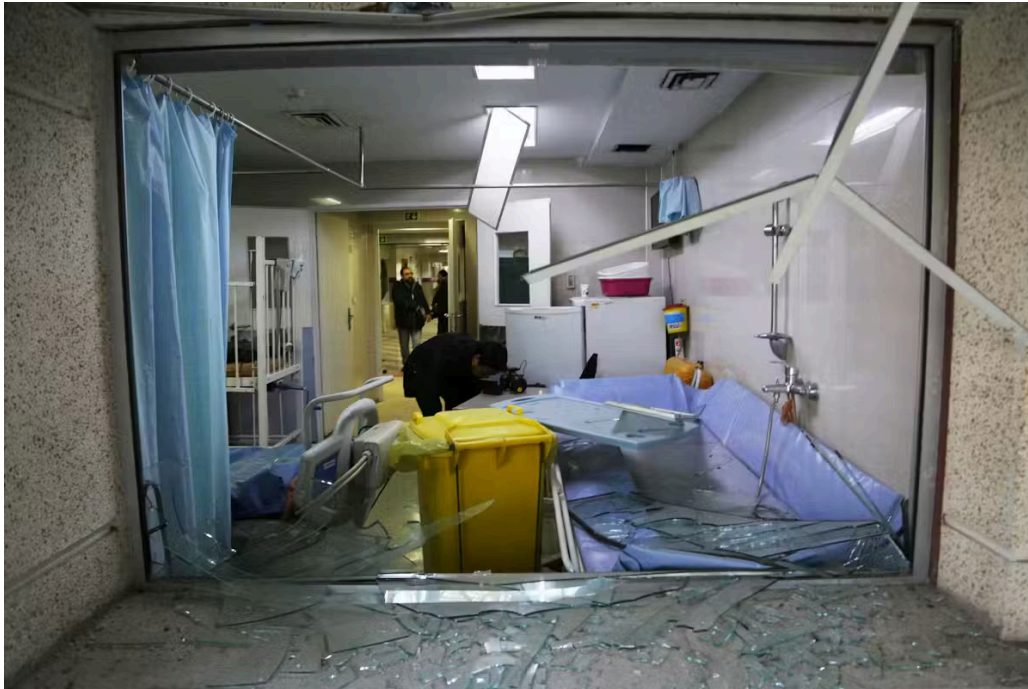
Damage caused by US and Israeli attacks on Shahid Motahhari Hospital in Tehran. Anadolu/Getty
